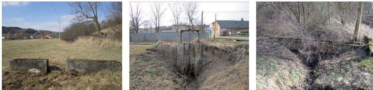
Figure 4 A setting device at none exist drive in 2017 (on the left), Example of a drain in 2017 (in the middle), An aqueduct across nameless watercourse in 2017 (on the right)
